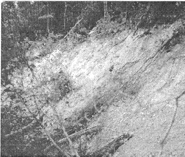
pic; a section of the top of the landslide; the vegetation above the embankment has not been disturbed, below it, vegetation has been swept away with the soil.
