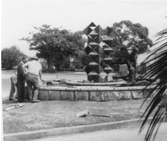
Construction of the Griffin Memorial Fountain in 1965. Note the crystalline shapes in freeform nodules of copper. Photo: Harry Fox
